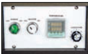
Tunnel Control Panel
